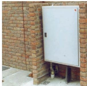
Six meter cabinet
