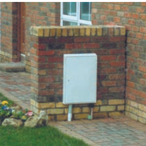
Domestic meter box
